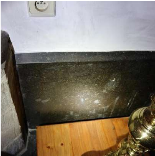
Barst in wand
