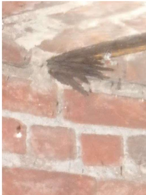
water in de kelder
